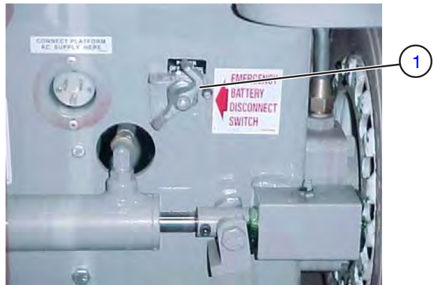
Figure 2-2. Emergency Battery Disconnect Switch
